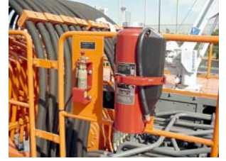
RED LINE HP Installed on Truck 03.jpg
